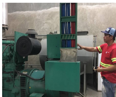
BSP Generator Set
